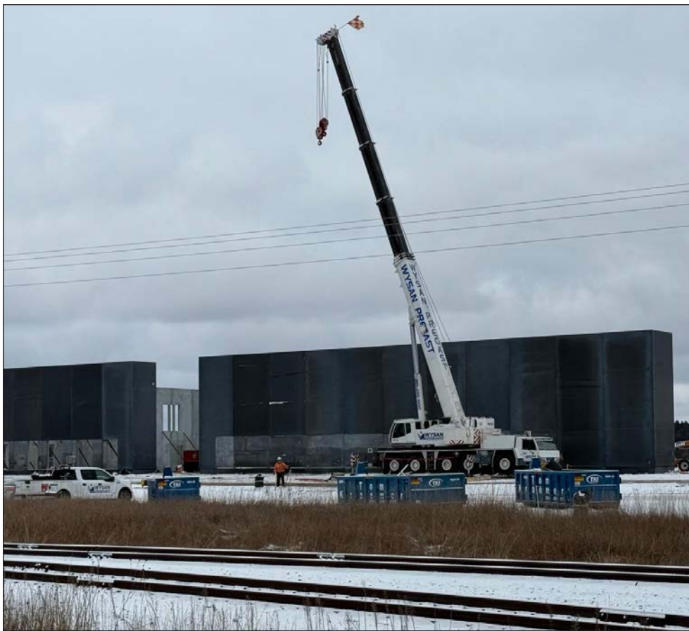
Construction workers have placed a few walls at the new site for the Minnesota Military & Veterans Museum. The museum is on 32 acres along Minnesota Highway 371.
